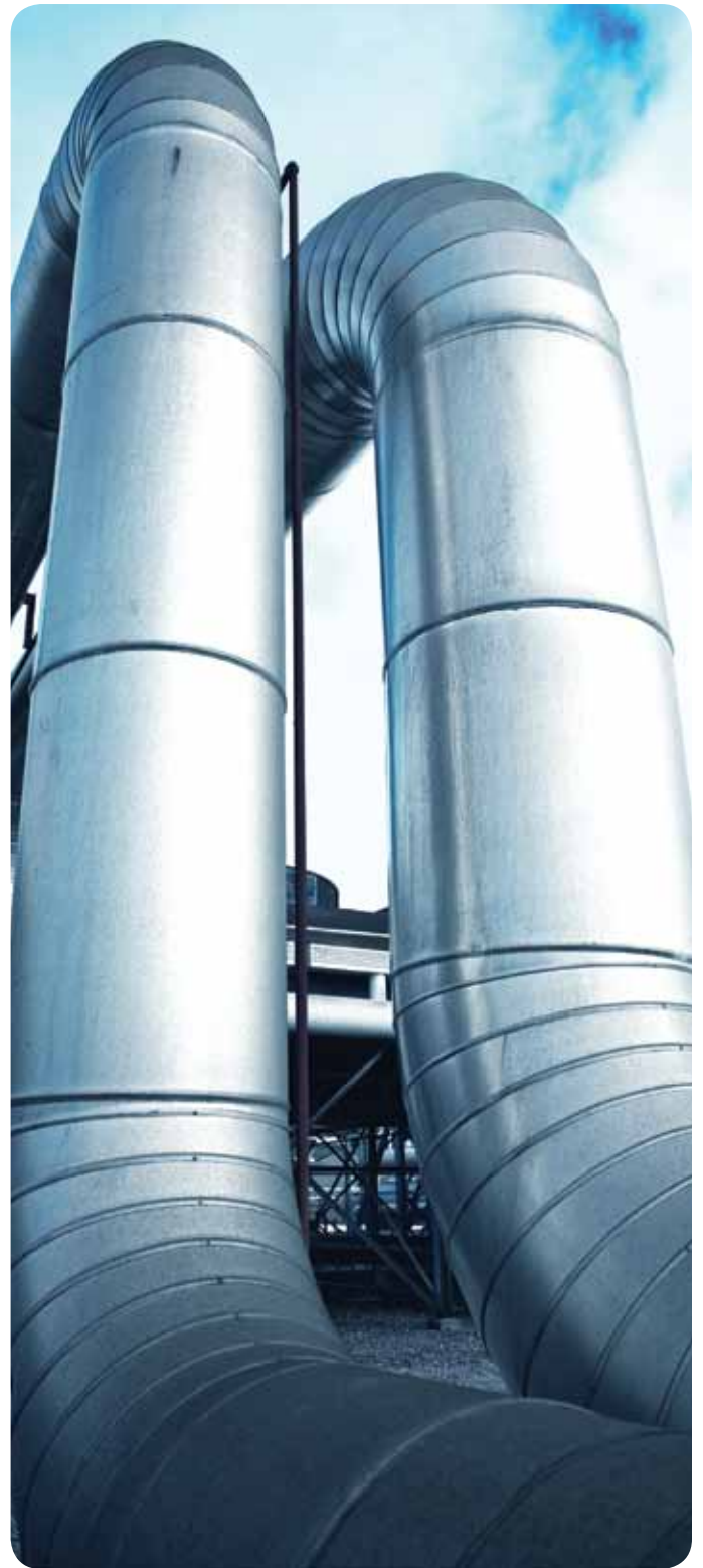
Completed in May 2010, the 140MW Nga Awa Purua Geothermal Power Station houses the largest single shaft geothermal turbine in the world. Nga Awa Purua is one of several joint ventures between electricity generator Mighty River Power and the Tauhara North No. 2 Trust.
