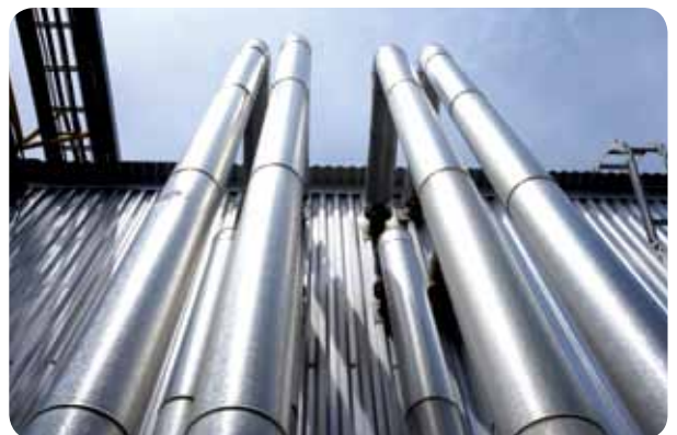
Silver Fern Farms' Finegand meat processing plant in Balclutha is turning sludge from waste water into a valuable biofuel, reducing the company's CO 2 emissions by 9,500 tonnes per year. The company aims for best practice in environmental stewardship and industry innovation.
